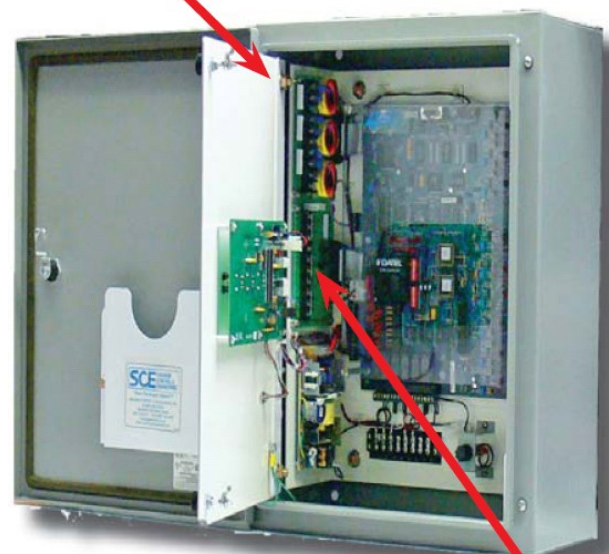
6PTP2 Potential Transformer Interface
